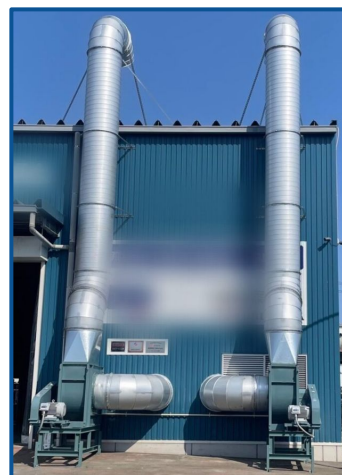
Exhaust fans and vent
